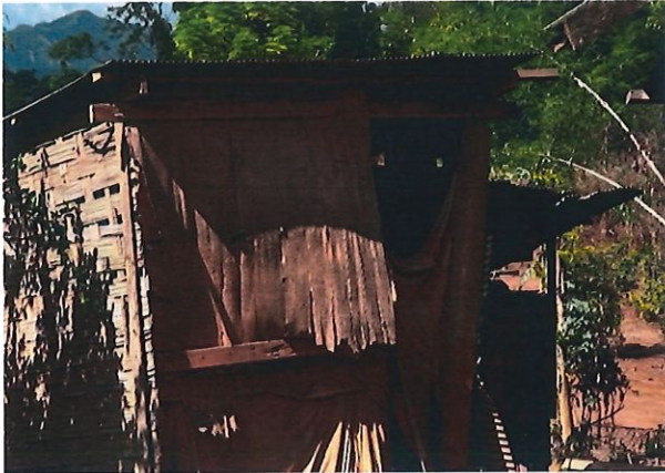
Figure 10: Many of the latrines are not usable, as they are either damaged or in need of extensive cleaning
