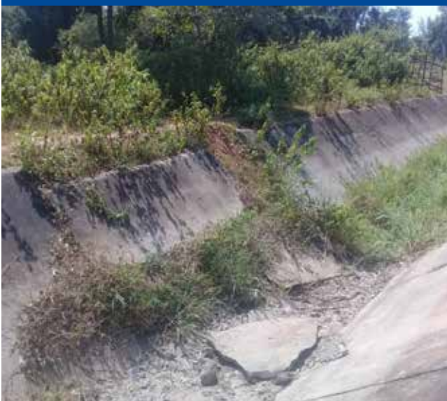
Damaged irrigation system in Khammuane Province.
