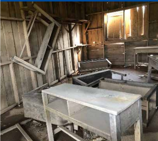
Destroyed classroom at Mahaxay Primary School in Mahaxay District, Khammuane Province.
