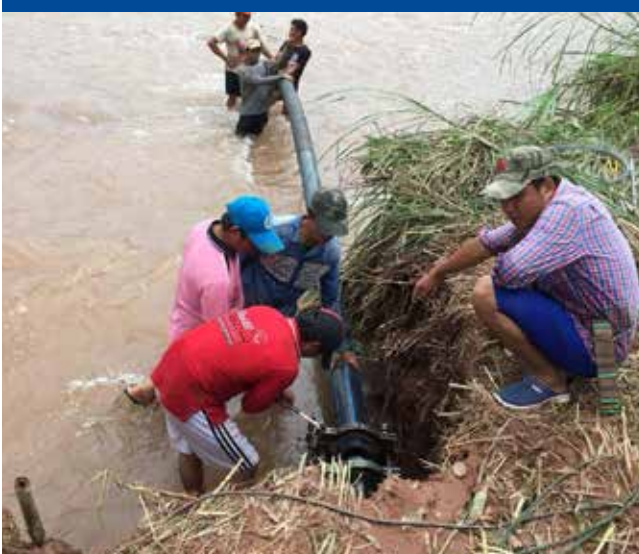
Nam Papa team of Beng District, Oudomxay Province, carries out emergency repairs to damaged urban water supply systems.
