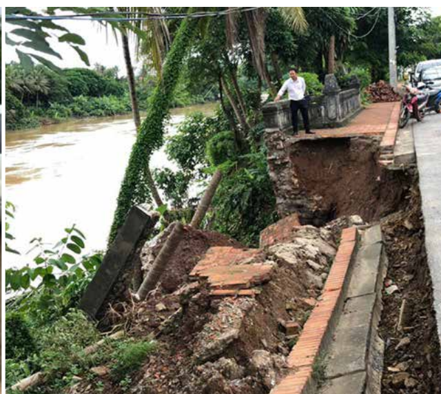
Damage to slope protection of Nam Kham River, Kili Village, Luangprabang Province.
