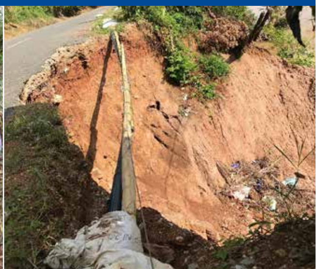
Damage on mainline distribution network of Nam Papa in Ngoy District, Luangprabang Province.
